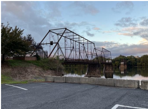
Bridge over the Susquehanna at Harrisburg that once carried the trolley tracks. Span was dropped by ice.
