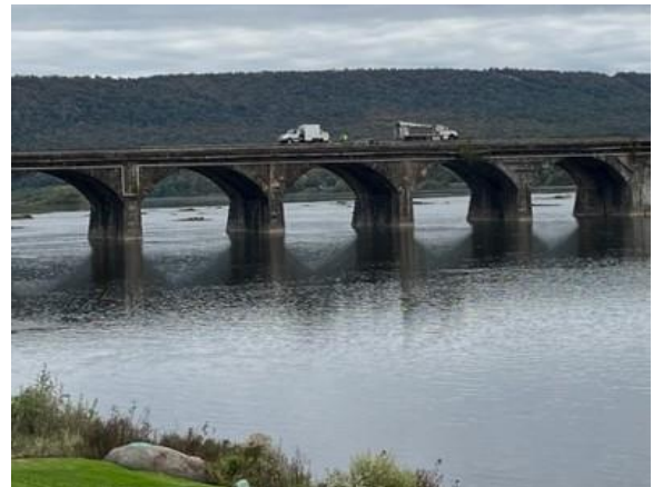
Hi-rail truck on the Rockville Bridge. They were building up a worn frog with welding.
